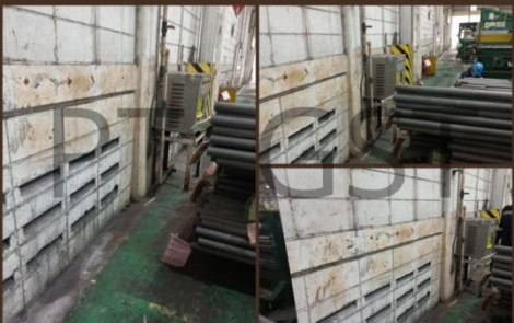
Cover Blower Boiler Room Draw Bench
