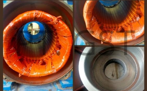
REPAIR MOTOR (BALANCING IMPELER)
