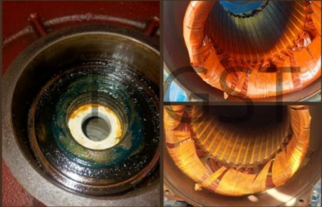
REPAIR MOTOR (BALANCING IMPELER)
