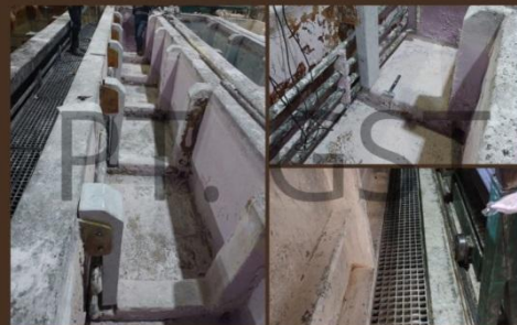
Front Stop FRP Grating and Stopper Phosphate Pickling Tank
